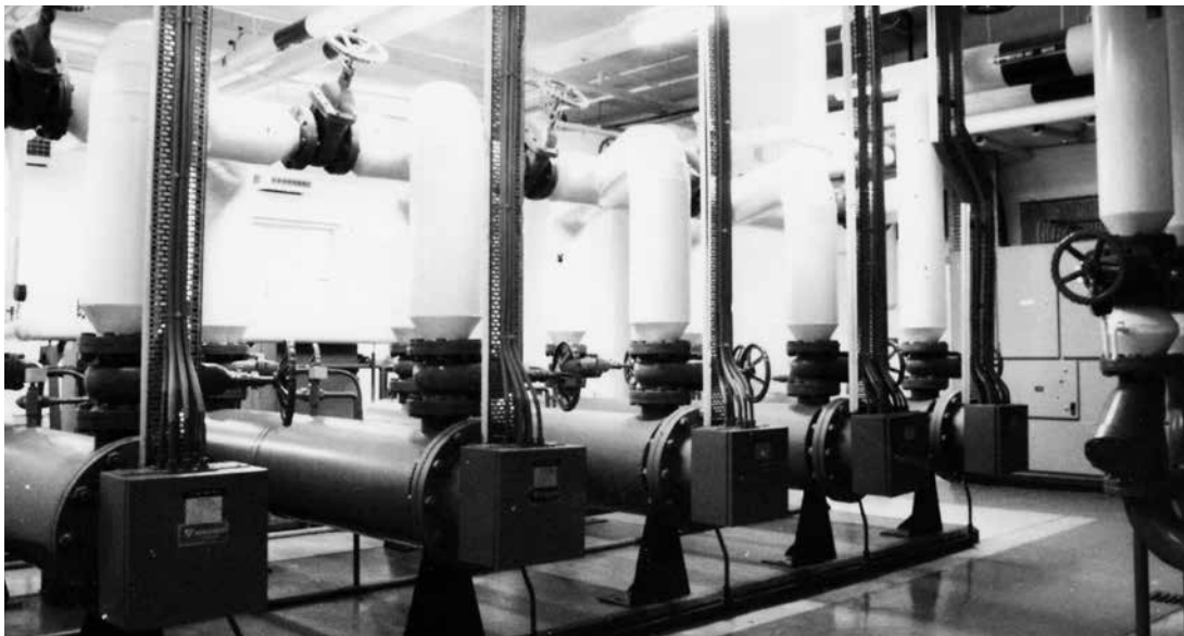
Electric boilers, c.1985.
